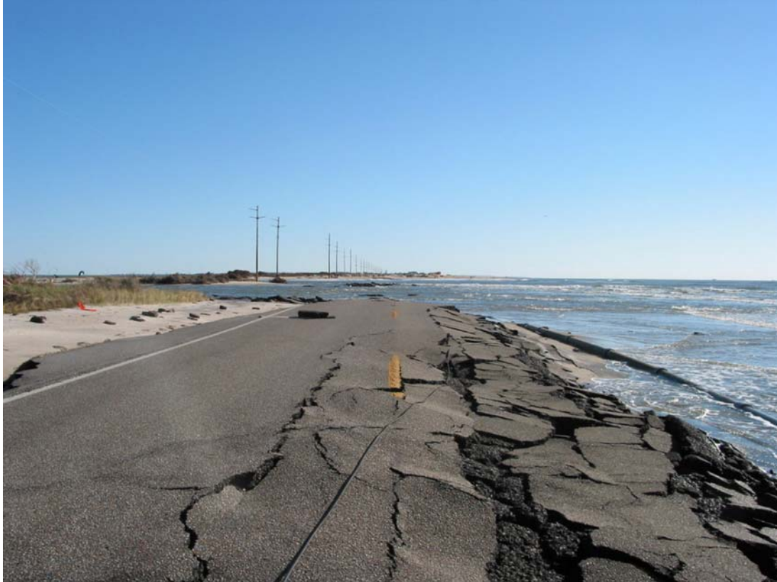
Figure 4. Photograph illustrating the debris within the central portion of the breach. Asphalt from NC12 and broken utility lines covered extensive areas (looking northeast).
