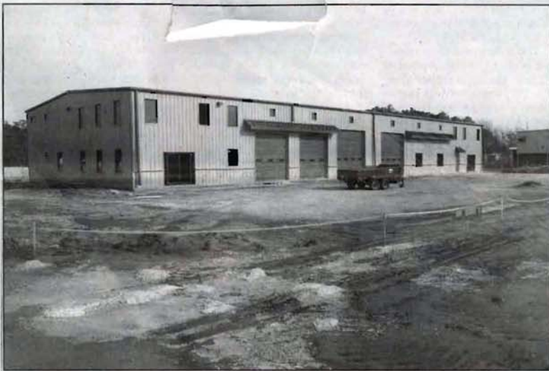
Geodynamics is building in the county-owned industrial park in Morehead City this 10,000-square-foot, two-story structure with 2,500 square feet of office space plus more than 1,500 square feet of shop space and boat storage. (Mark Hibbs photo)
